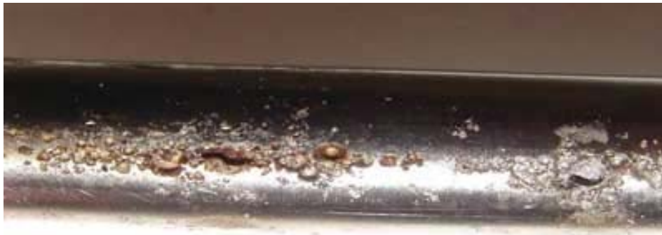
Figure 1. Pitting corrosion in stainless steel pipeline.
