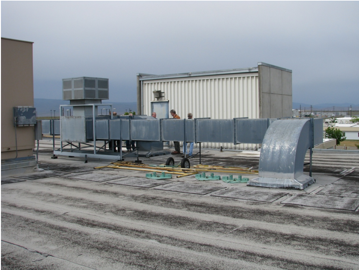
Figure 3. Existing HVAC unit on 2750E Building.
