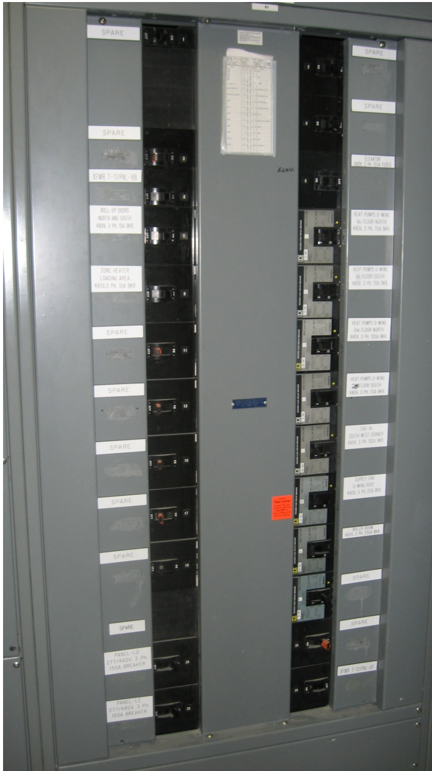
Figure 13. Electrical panel for upgrade.
