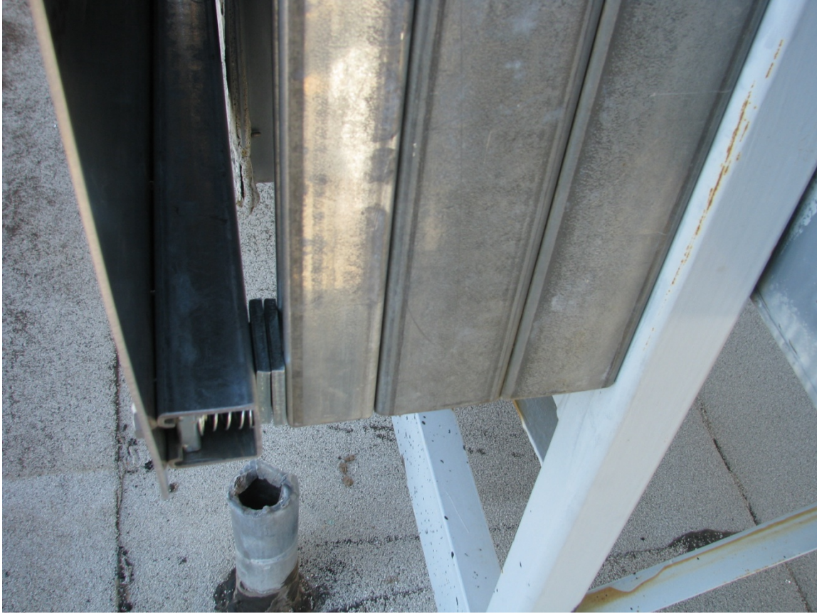
Figure 12. Side view of control enclosures.
