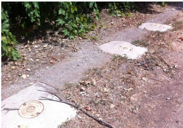
Figure 4. Example of Adjacent Flush Mount Well Series in Industrial Site 'L'
