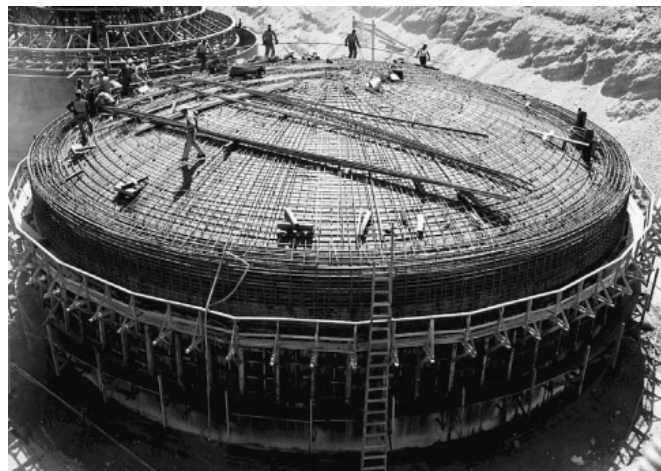
Figure 6. Construction of reinforcement bar for tank dome in BX farm. Taken from [1]
