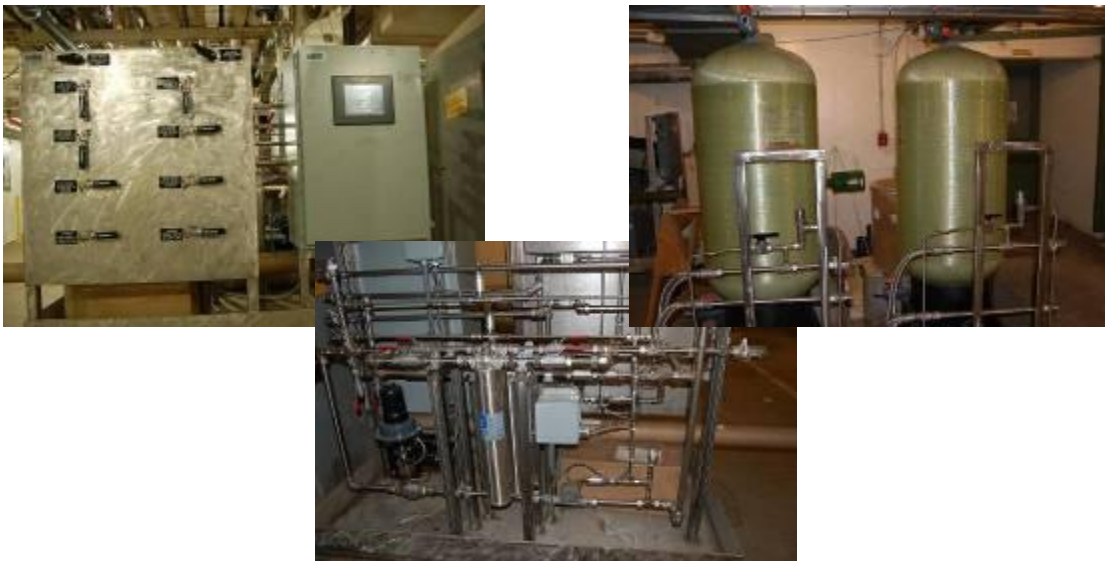
Figure 2. Mercury treatment system located at Building 4501, Sump I.
