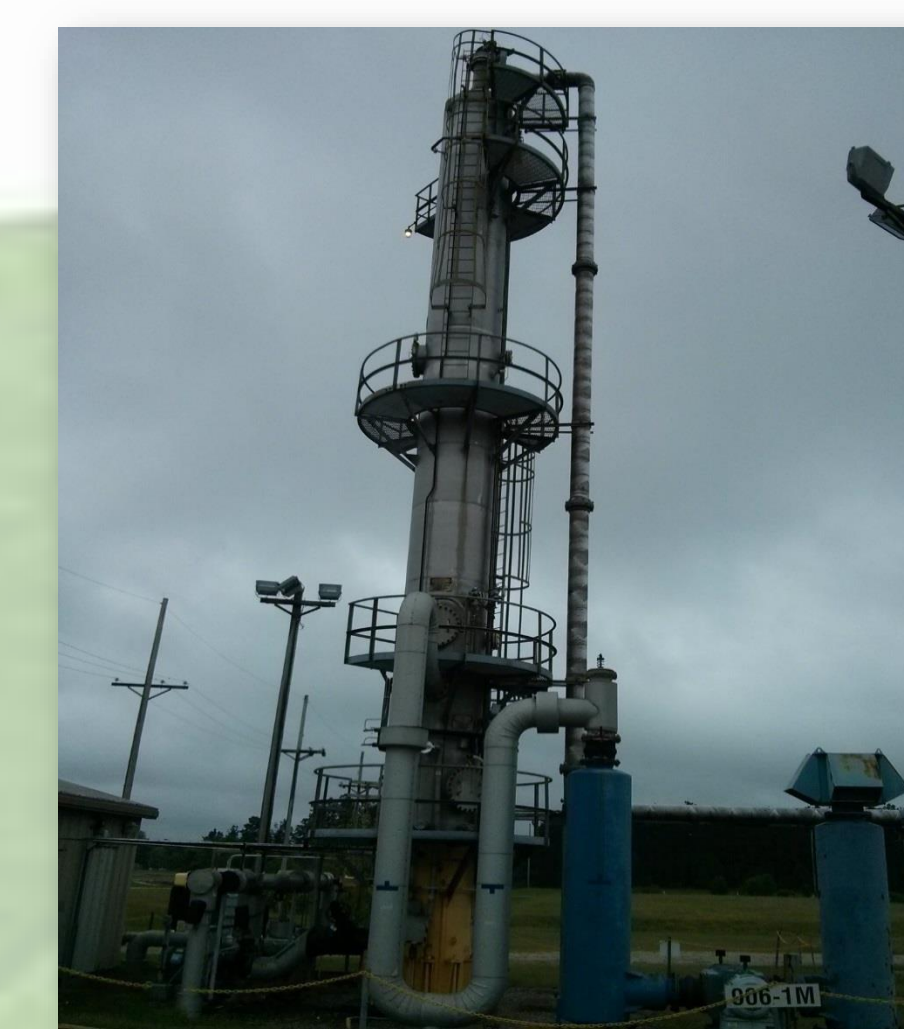
Figure 5. Photograph of the full-scale M1 air stripper at M-Area at SRS.
