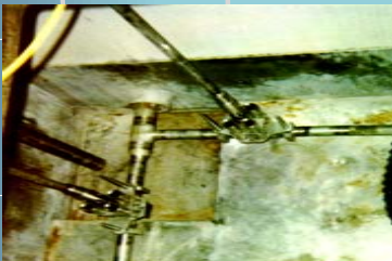
A Tank Farm plug occurred at the Idaho National Lab because valve on 3" pipe did not open fully (globe valve not ball valve). Solids clogged the restricted passage. The globe valve was removed and no plugging has occurred since that event.
