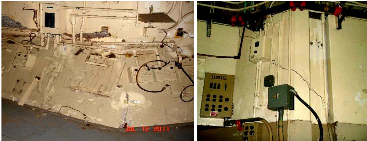
Figure 6. Interior cracking for LLNL Building 280.
