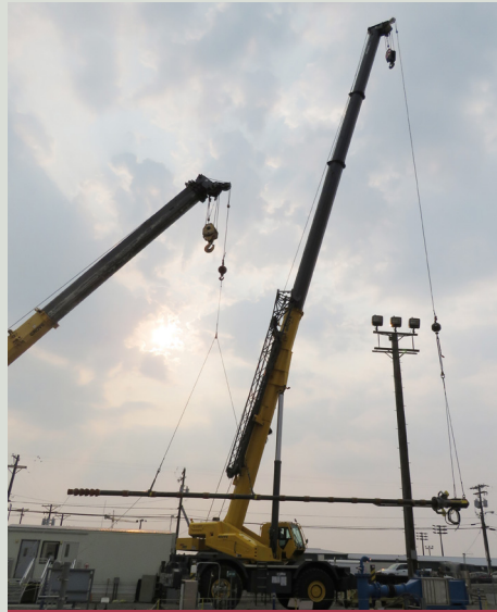
Workers use a crane to install the new feeder pump in Pit AW-02E. The feeder pump will support future Evaporator campaigns.
